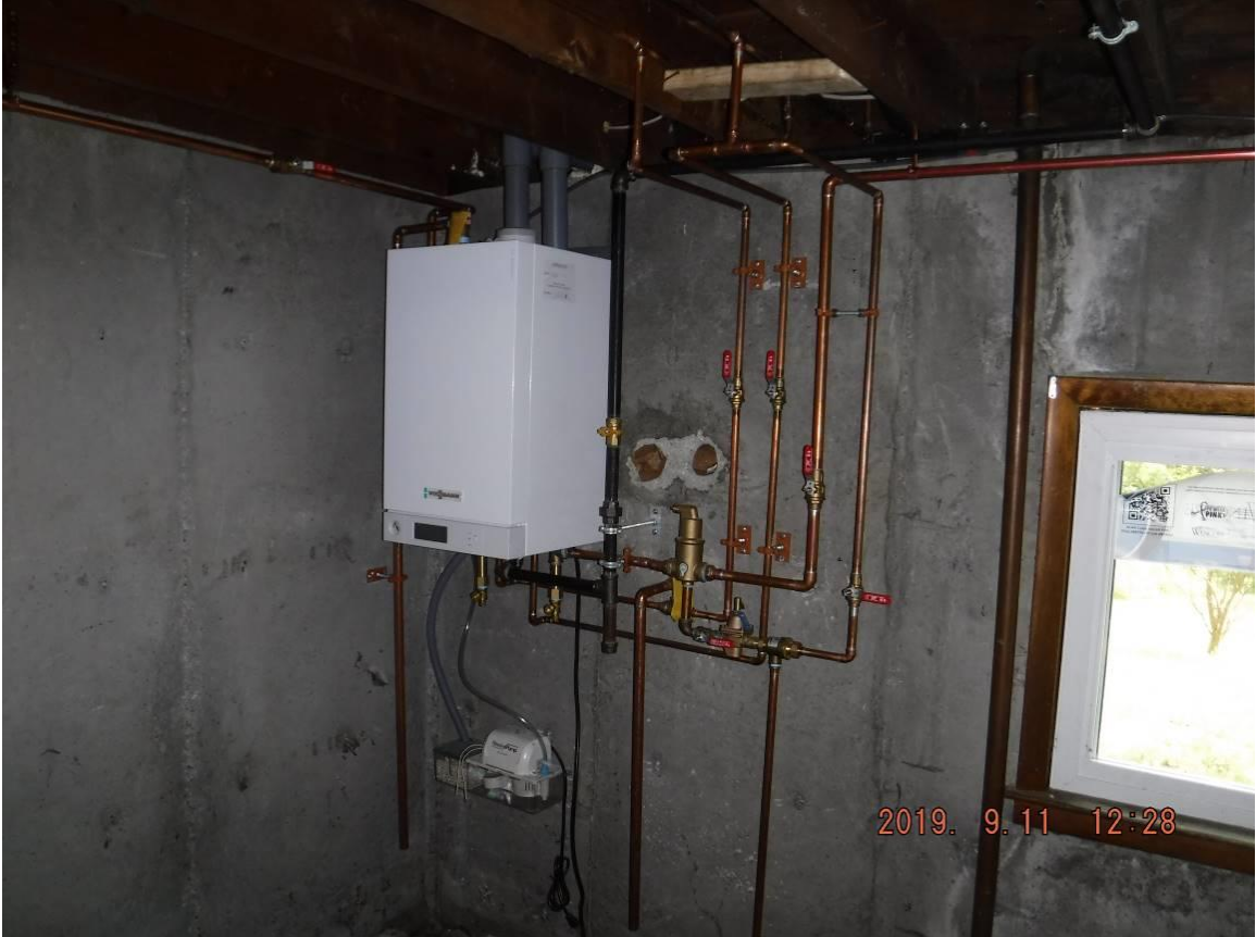
870 East St, Lenox MA – Photos new gas fired boiler and plumbing.
