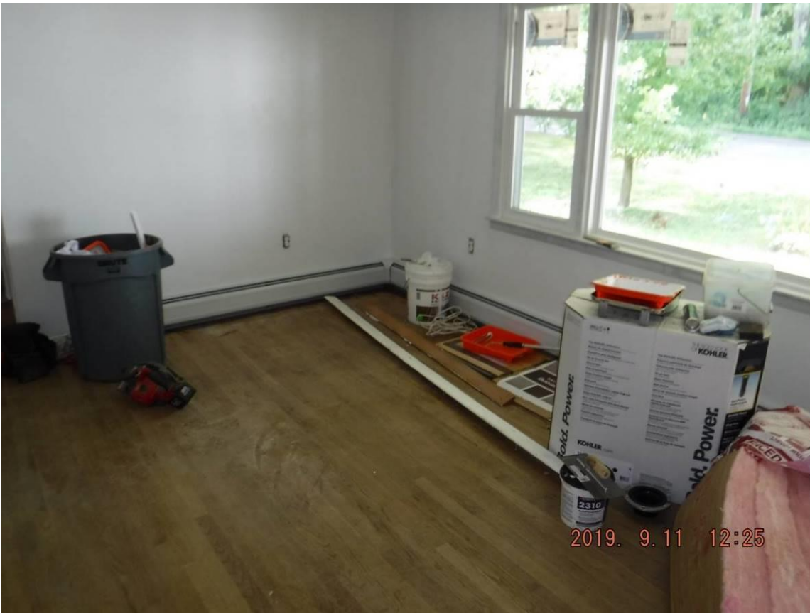
870 East St, Lenox MA – Representative photos of living room and bedroom with walls primed and new baseboard radiators installed.
