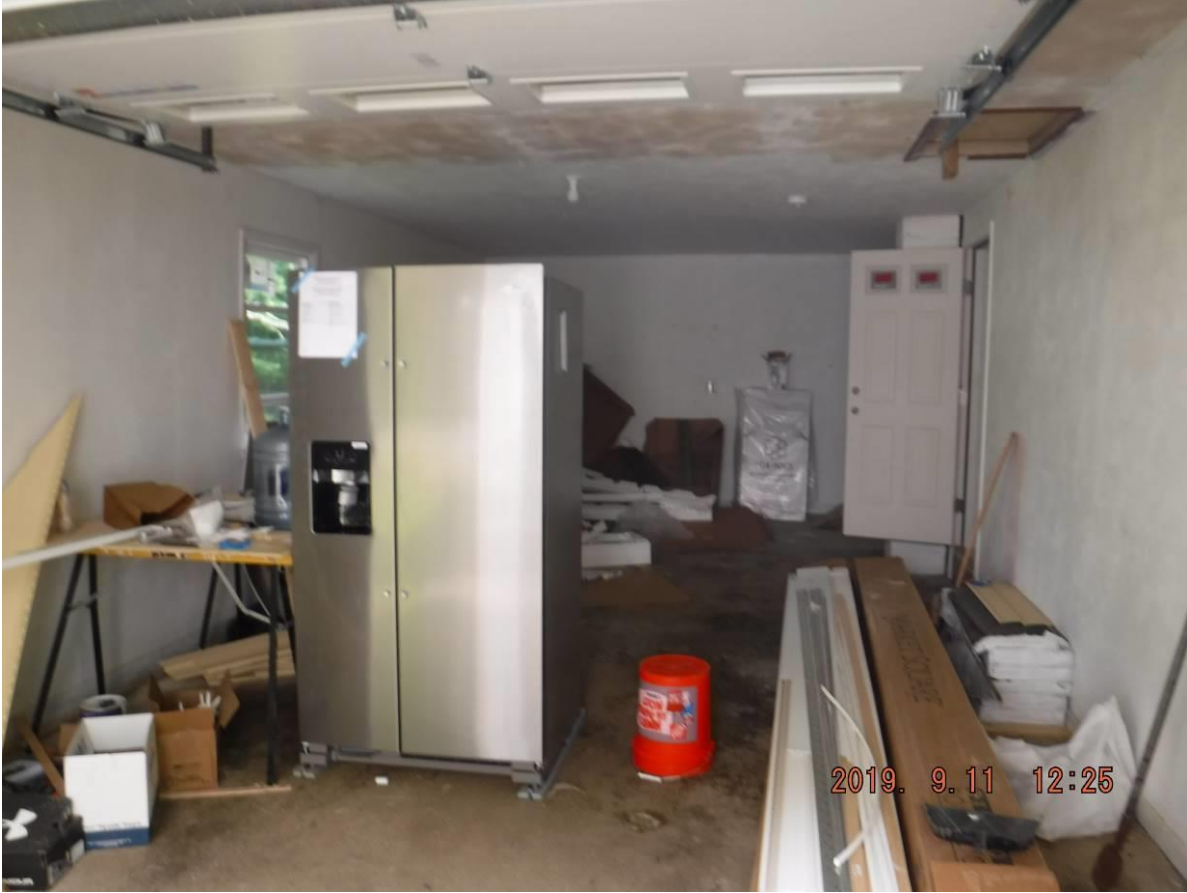
870 East St, Lenox MA – Garage with new refrigerator and materials (top) and back yard (bottom) marked out for new septic installation.
