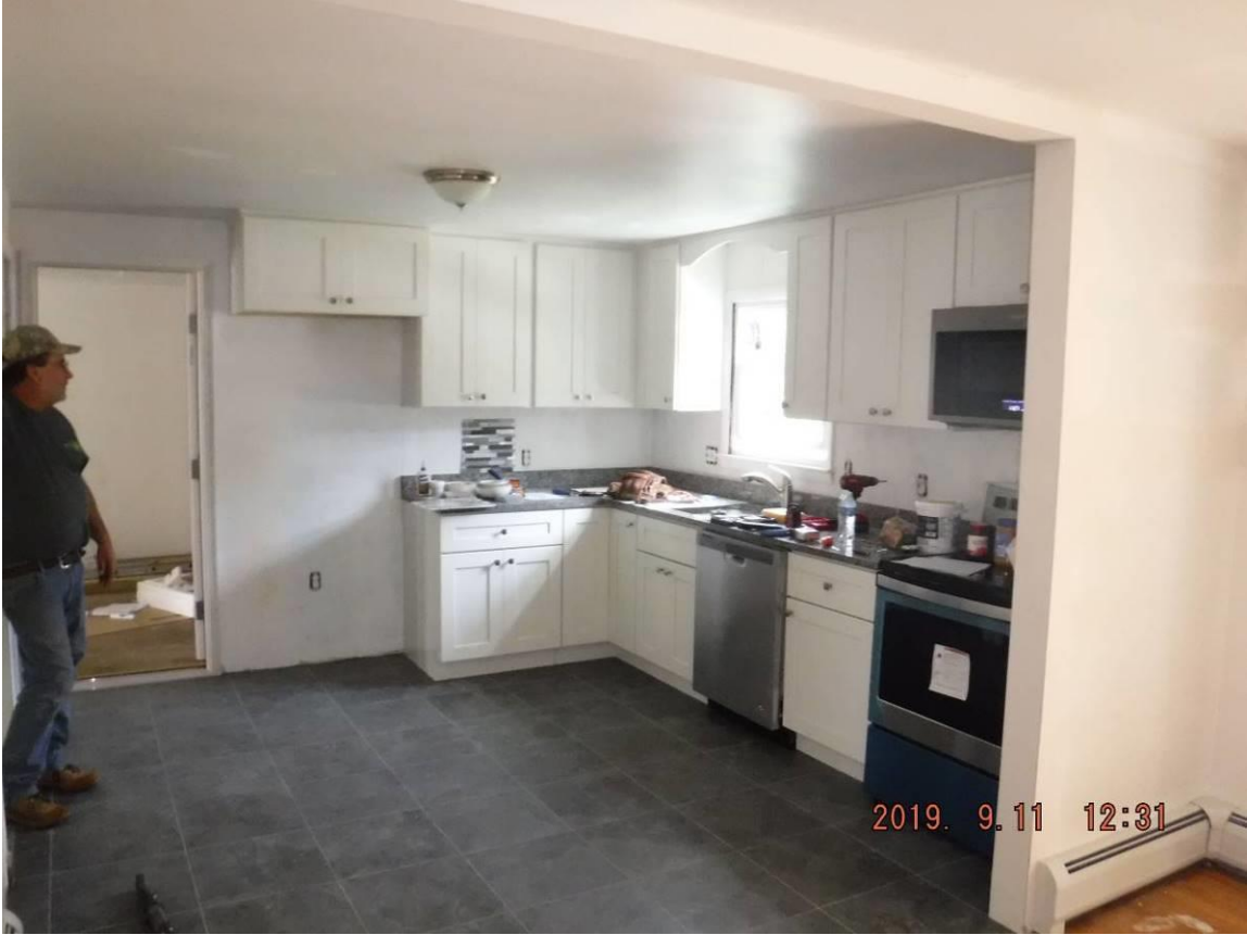
870 East St, Lenox MA – Photo's of kitchen (top) with new cabinets, flooring and appliances in progress and bathroom (bottom) with new flooring, bathtub, insulation and radiator.
